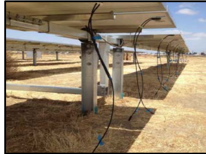
Dirt Inside Connectors
