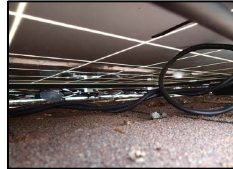
Wires Rubbing On Roof
